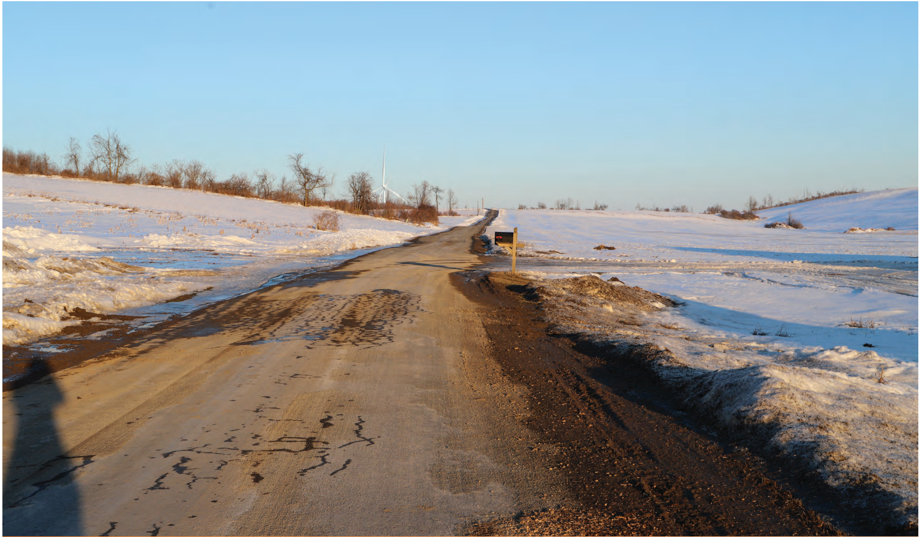
Photo 3 - Parmwood Rd. SIMULATED CONDITION
